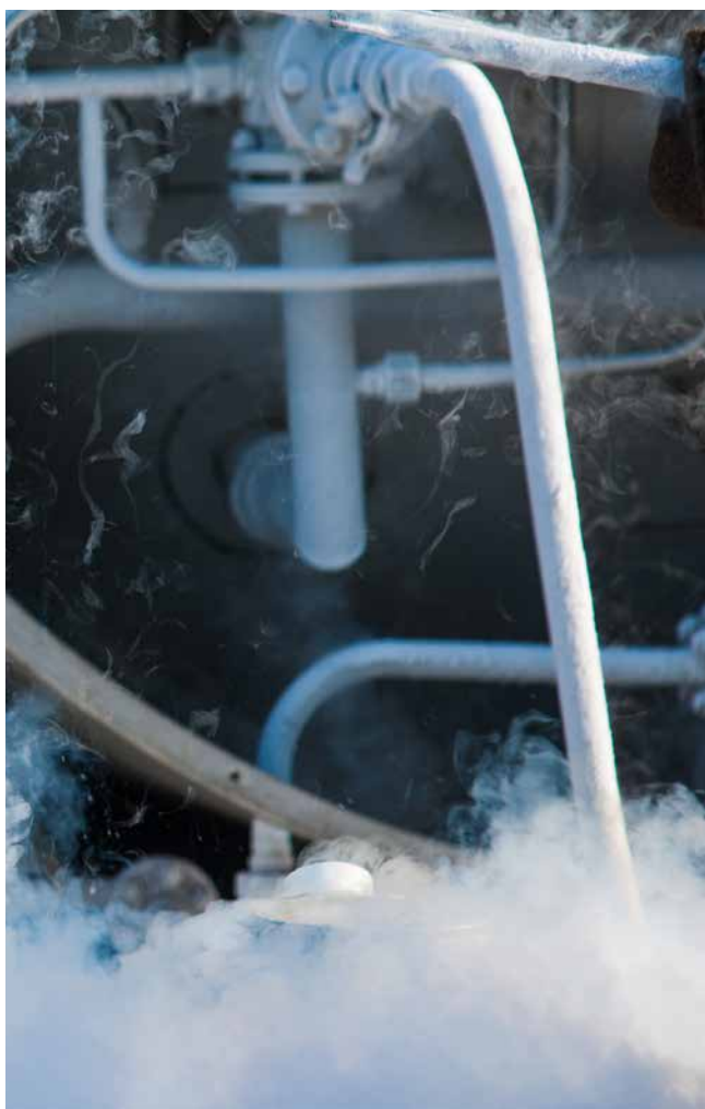
Axial split, between bearing pump (API BB3) operating on low temperature ethane application
